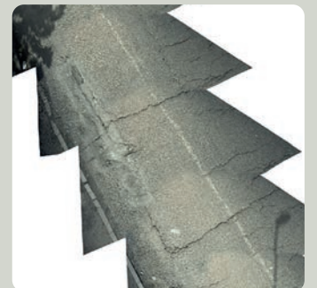
Orthomosaic showing poor road condition in TBC
