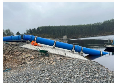
Survey data was used to help the dive team to position infrastructure
