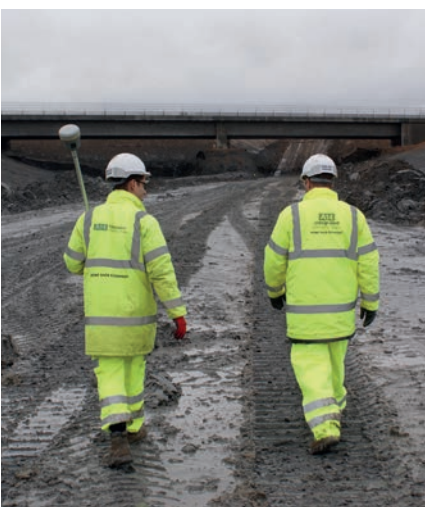
▲ The Trimble R10, first adopted on the M1 improvement scheme in Rugby and now used daily on the A14 site
