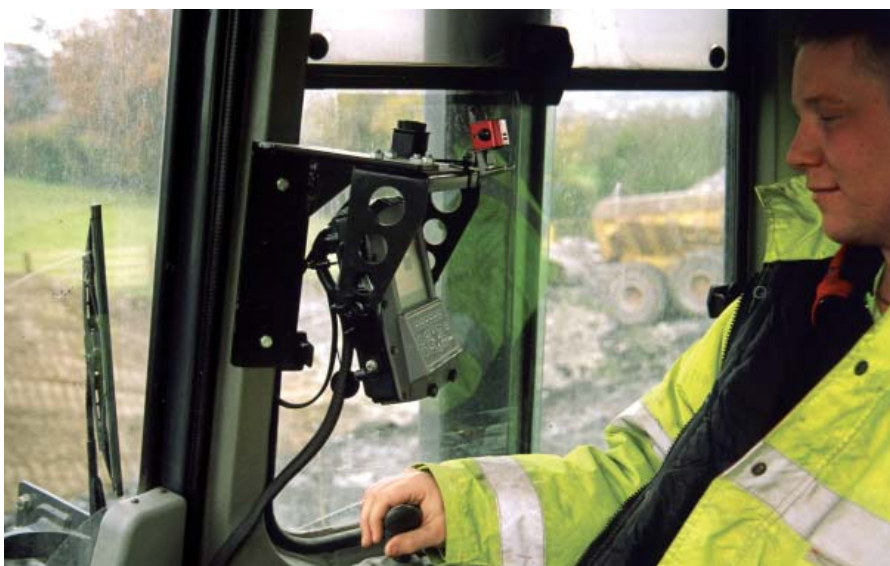
▲ "There is no engineer setting out or putting stakes in the ground because everything required to grade is on board the dozer"
