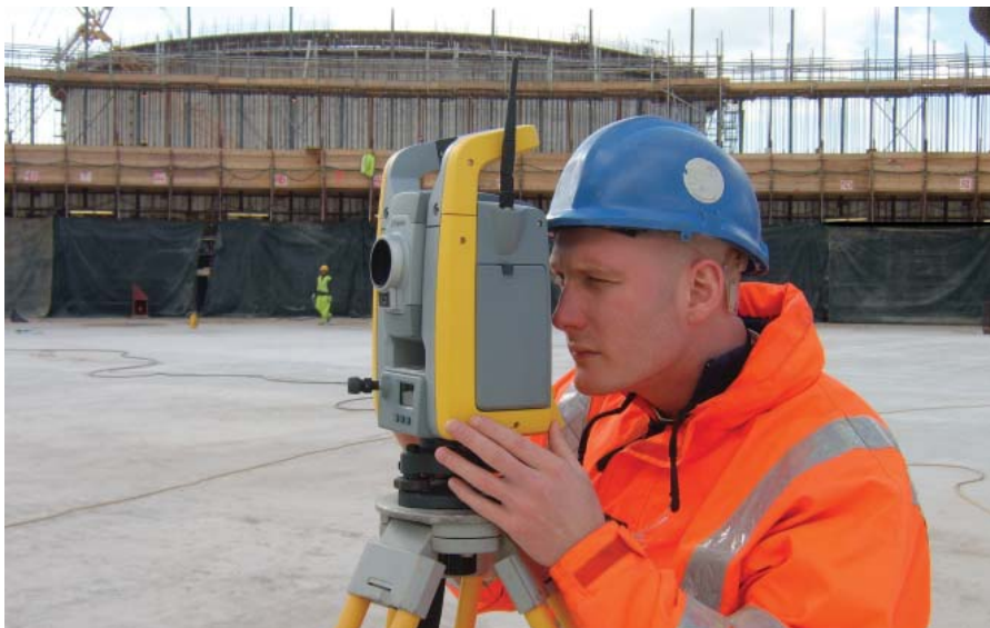
▲ TWC Surveyor Jim Garside with the Trimble S6 in the centre of Tank 5 with Tank 1 in the background
