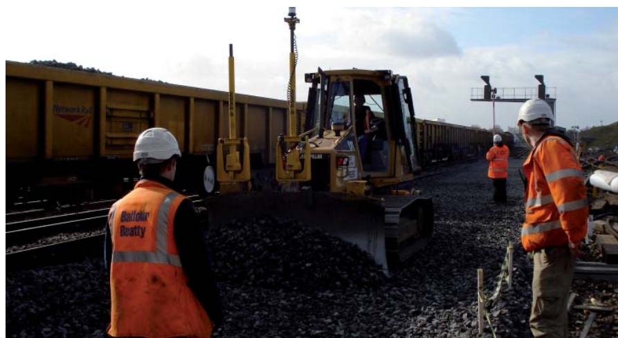
▲ Millimetre accuracy - a single electric mast with an active target prism centrally mounted on the blade of the dozer and a slope sensor calculate blade tip position of the machine
