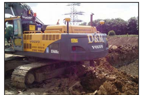
Dual Trimble MS990 integrated GPS receivers were mounted onto the back of the excavator
